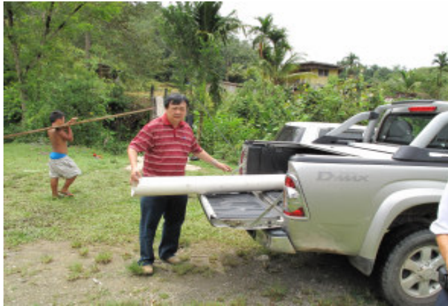
PP Peter Yapp hard at work unloading pipes and other hardware at Kg. Timbangoh Laut, Penampang for the Gravity Water Feed project.
